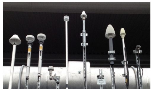
GPS antennae placed too close together
