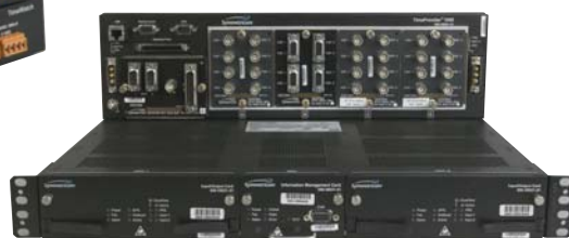
TimeProvider, the latest access layer sync equipment from Symmetricom
