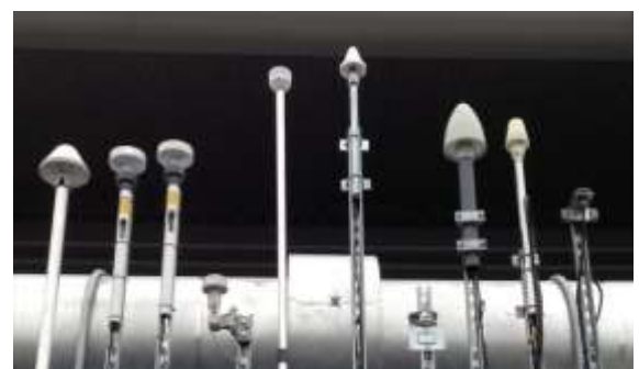
Antennas placed too close together
